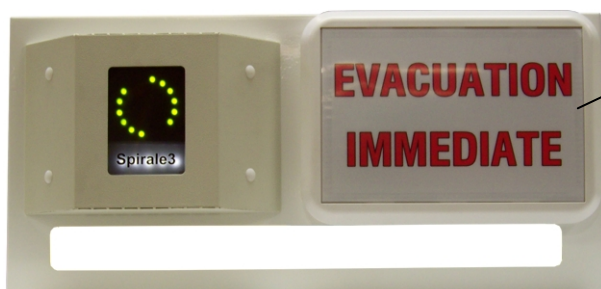
"Immediate evacuation" lighting sign, actuated by the control unit
